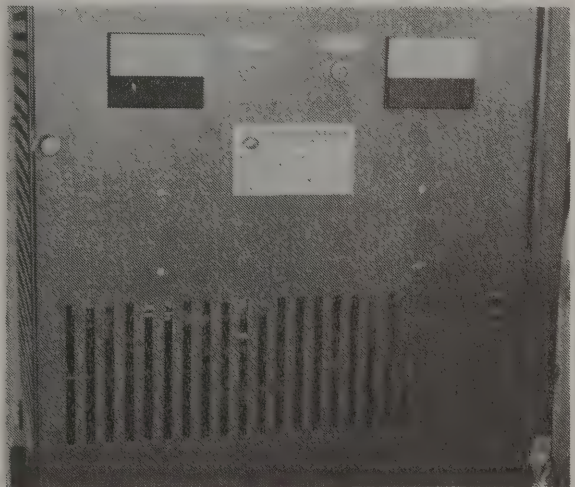
The Gemini inverter which took electricity from the Hydrowind and fed it into the P.E.I. power net on opening day — "running the meter backwards." The man from the power company advised, "Let me know before you do that again. Your electricity has too much noise in it still."
